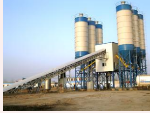
Batching Plant 1 Nos. 30 M 3
