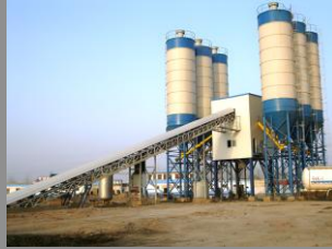
Batching Plant 1 Nos. 30 M 3
